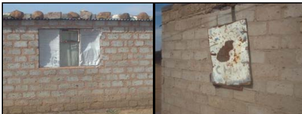
Figure 5 Non-functioning windows that have been covered
